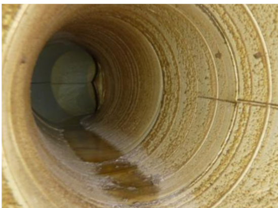
Exhaust duct without ozone cleaning system
